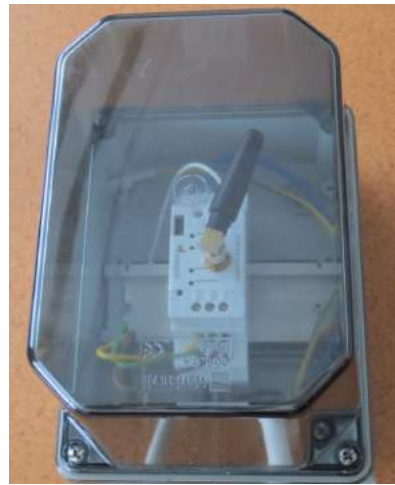
Meter installed in protective box Photo from Pacific Northwest National Laboratory
